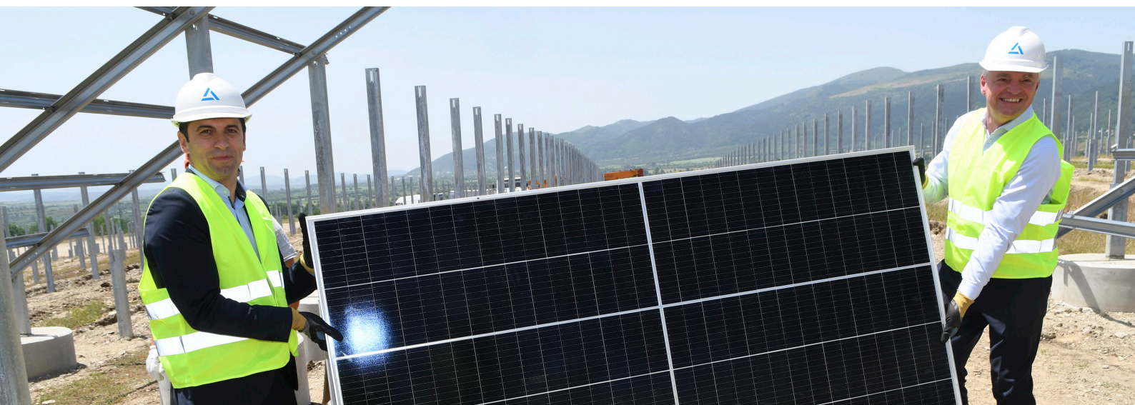
Kiril Petkov, Ministry of Economy in Bulgaria, and Roland Harings, Aurubis CEO, came to Pirdop, Bulgaria, for the construction kick-off for the largest internal company photovoltaic plant on June 24, 2021.
