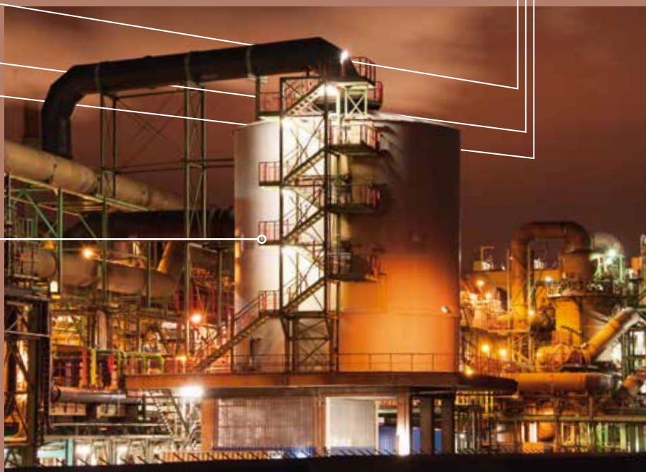
The renovated off-gas cleaning facility for the sulfuric acid plant in Hamburg is one of many examples of how we approach the increase in requirements for technical environmental protection.
